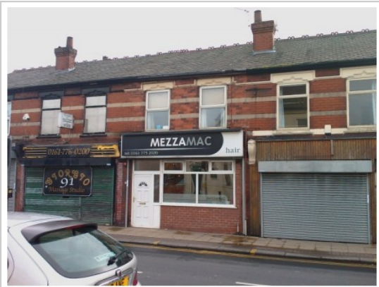
Above: A row of shops before refurbishment. the shop fronts do not relate to each other or to the buildings. In addition, the solid shutters detract from the streetscene.
